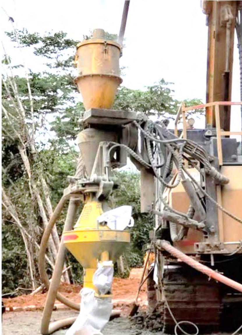
Figure 10.6: Rotary Splitter Attached to Metzke Cyclone
